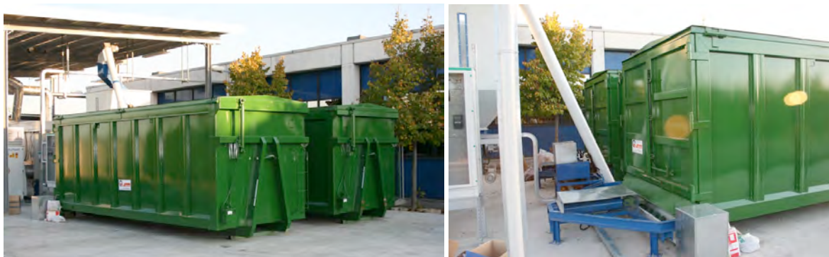
Figure 5 A plant with roll-on containers and container downloading system
